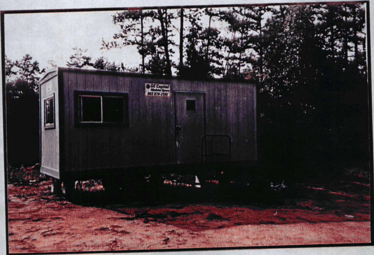
Original site trailer, an additional trailer was later placed along side of this one.
