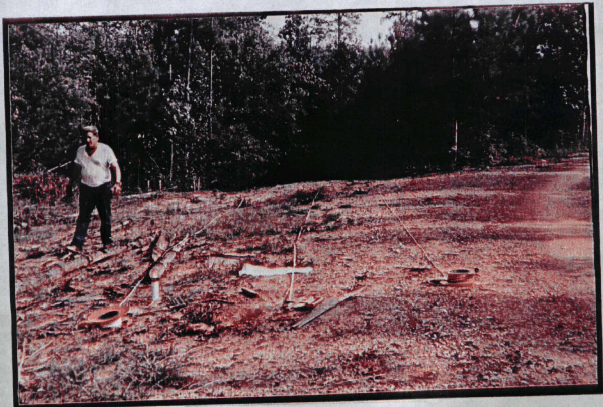
Laying out sweep lanes in lay down area for sweeping and clearing.
